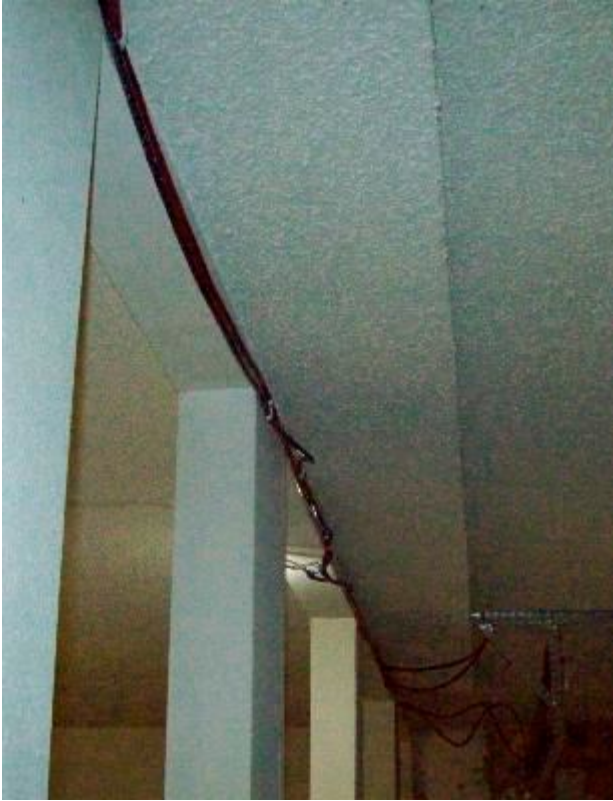
These are the 12 volt DC power lines I have in my basement
